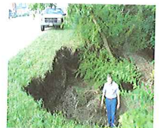
Erosion of drainage ditch along Airway Rd.
